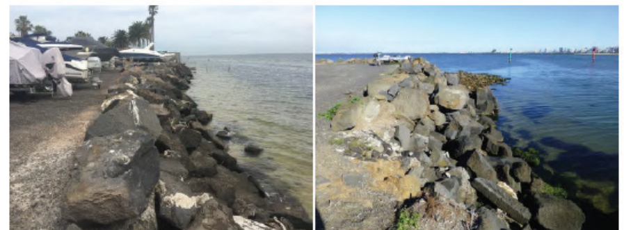
FIGURE 7-2 WESTERN SEAWALL: SEAWARD OF HARDSTAND AREA (LEFT) AND AT THE MARINE ENTRANCE (RIGHT)
